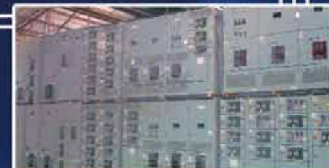
600V Class Switchgear Lineup
