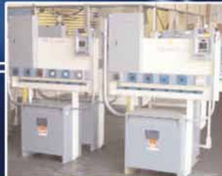
Temporary Power Transformer
